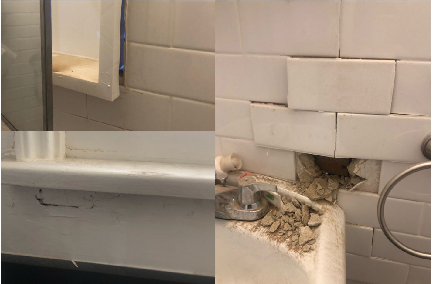
The impact of a 10-week construction project on a neighboring unit. The bathroom's vanity has fallen off, walls have extensive cracks, and tiles are dislodged, exposing the adjacent unit. The intrusion of dirt and the noise of incessant jackhammering exacerbates the problem.
